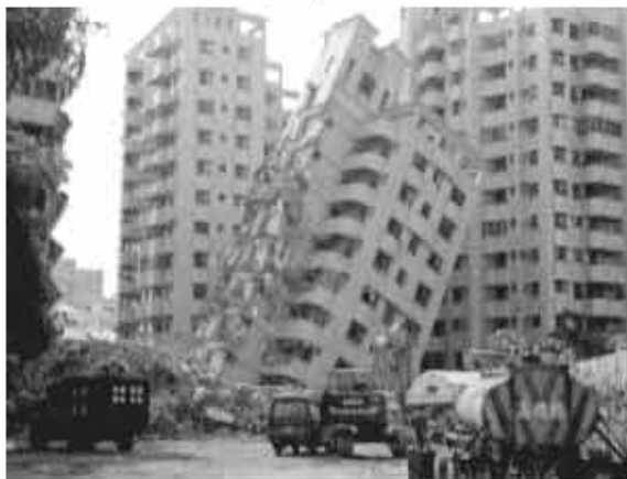
Fig. 14.3 : Building destroyed by earthquake
