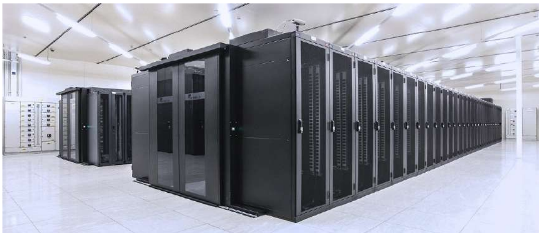
Photo of Bangladesh Data Center
